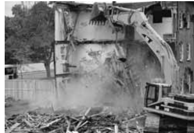
De-construction at a building on Sherbrooke St. in preparation for the CLSC move.
